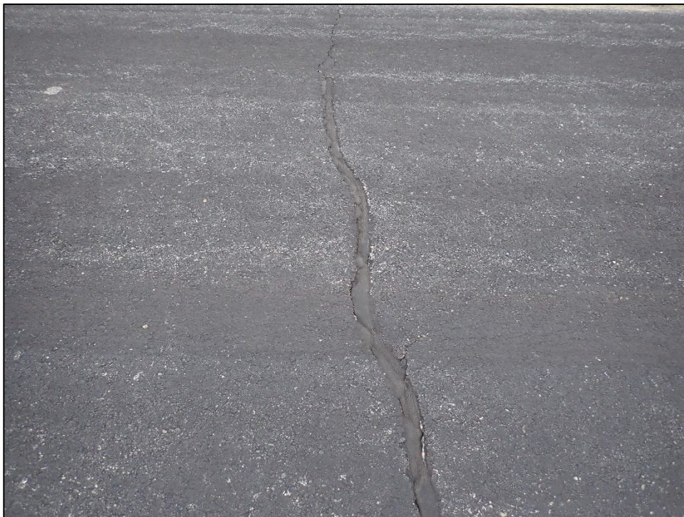
TW-05-08: L&T Cracking
